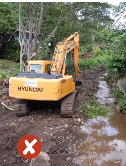
Working in the stream channel with no separation from stream flow.
