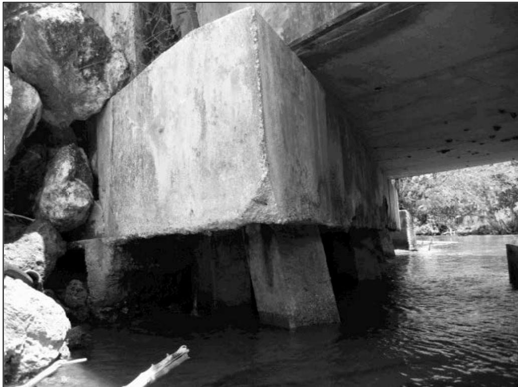
Photo 2 – Undermining of south abutment pile cap
