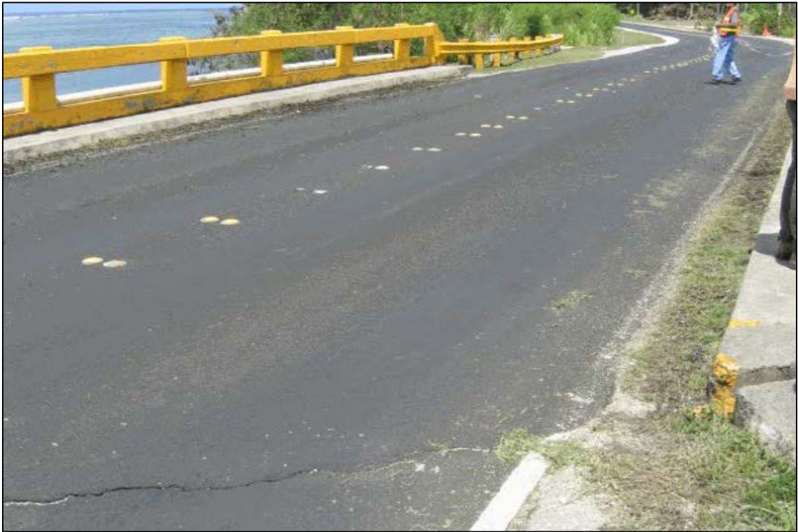
Photo 1 – Cracking demonstrating differential movement of the bridge
