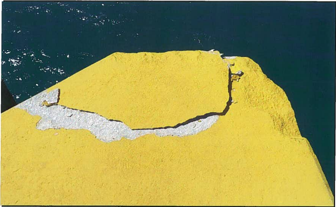
Damage to Left Side Corner Surface Deck at F-1 Dock Fender
