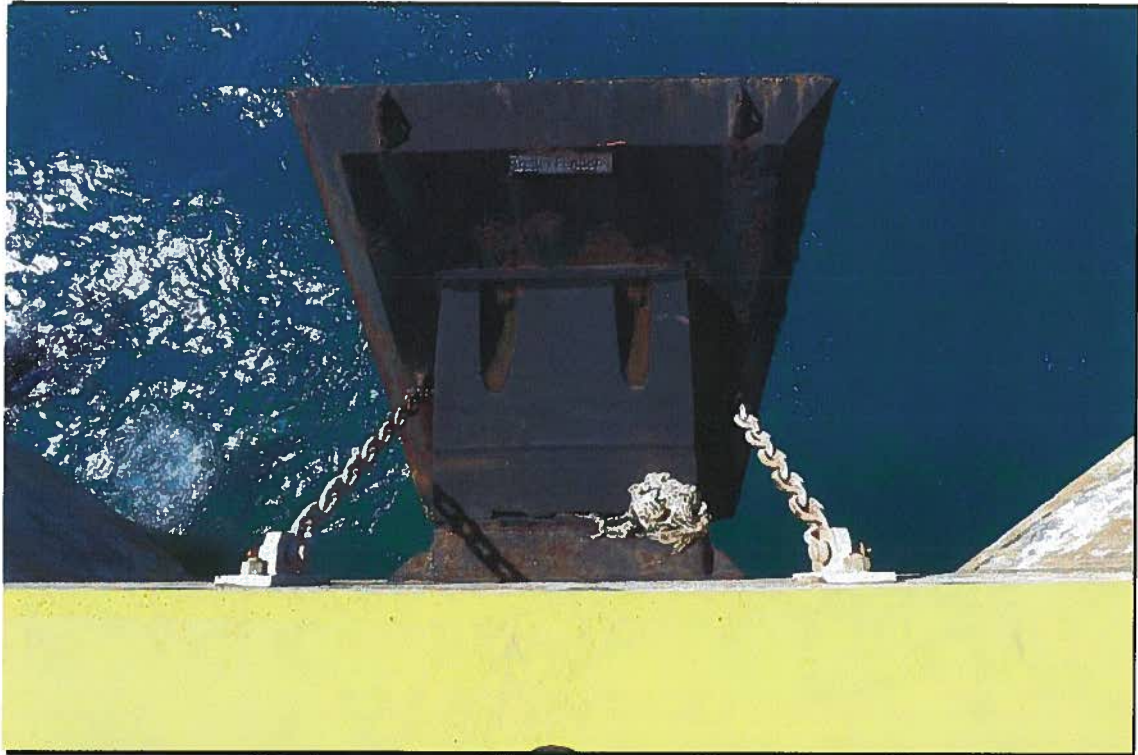
Damaged Fender System at F-1 Dock
