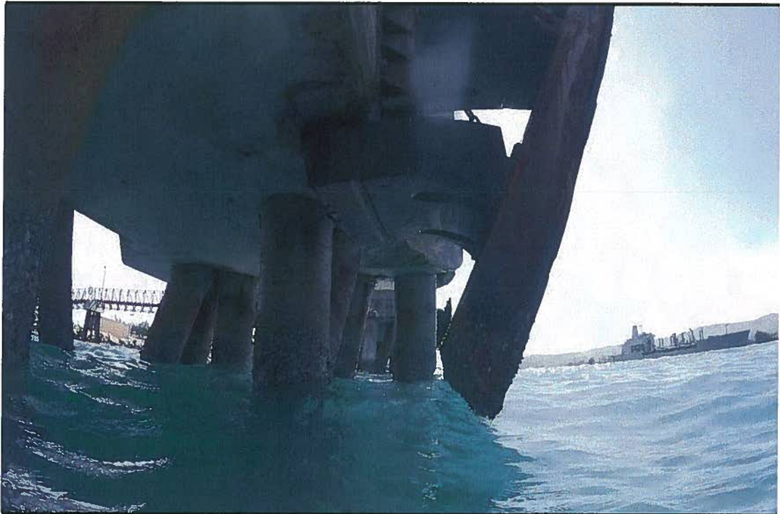
F-1 Dock Piles with Damage to Fender System
