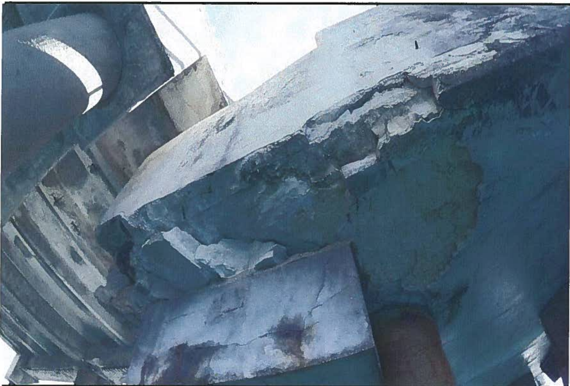
F-1 Dock Piles with Damage to Concrete Cap
