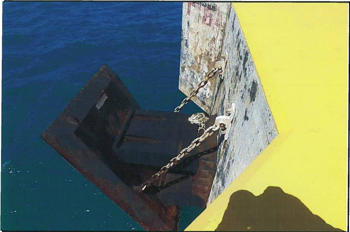
Damaged Fender System at F-1 Dock
