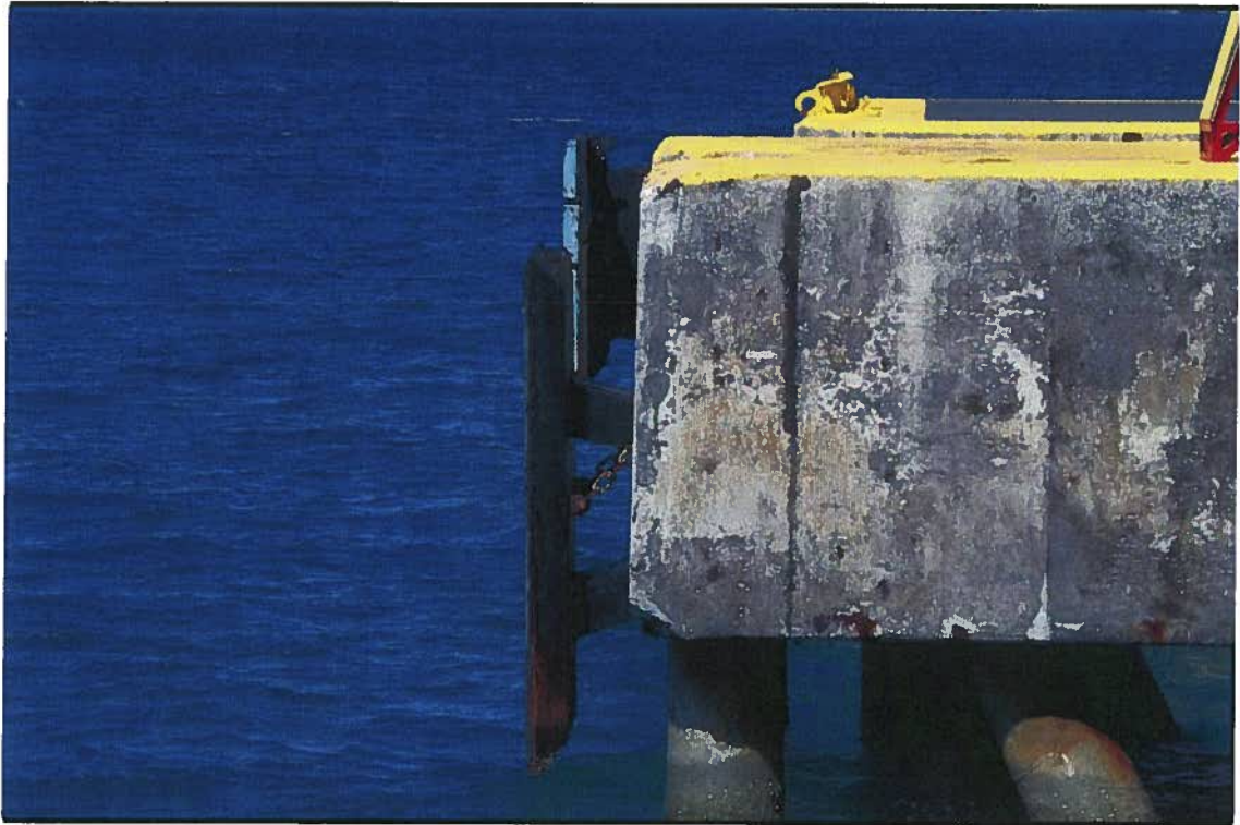
Far Left Side Fender System at F-1 Dock (Undamaged)
