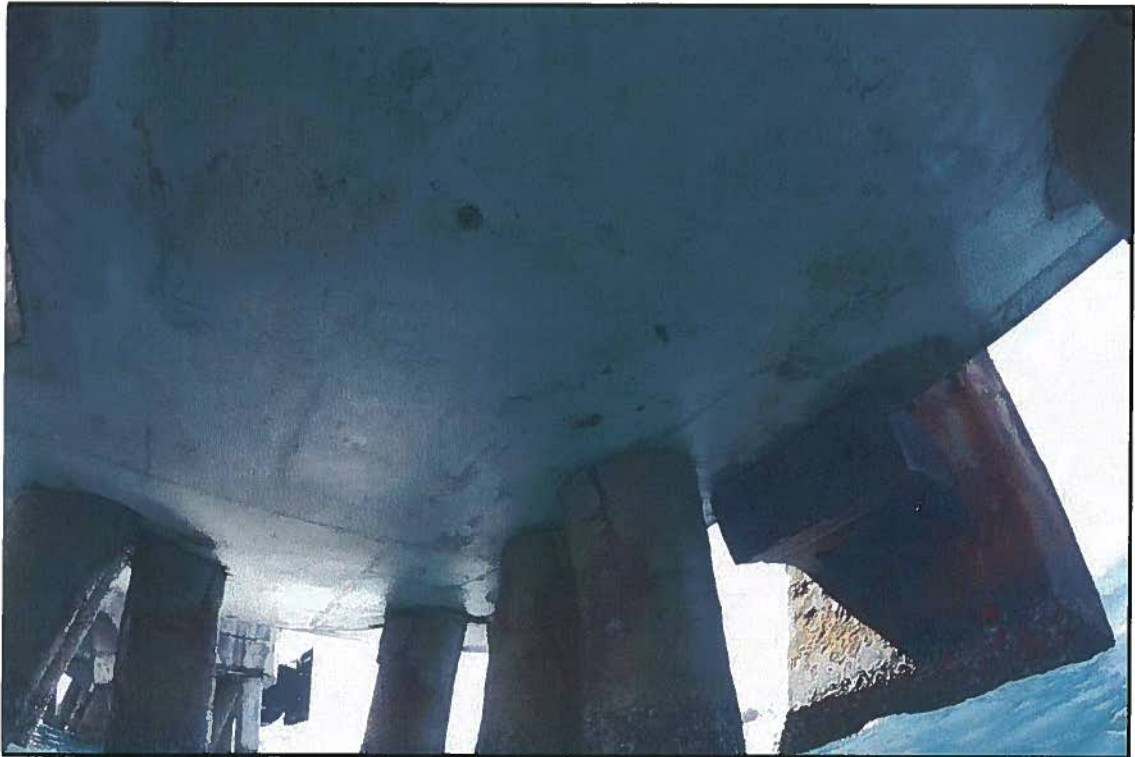
F-1 Dock Piles with Damage to Fiberglass Wrap and Fender System
