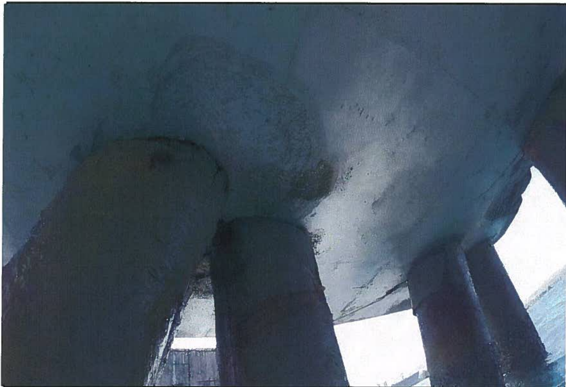
F-1 Dock Piles with Damage to Fiberglass Wrap and Concrete Cap
