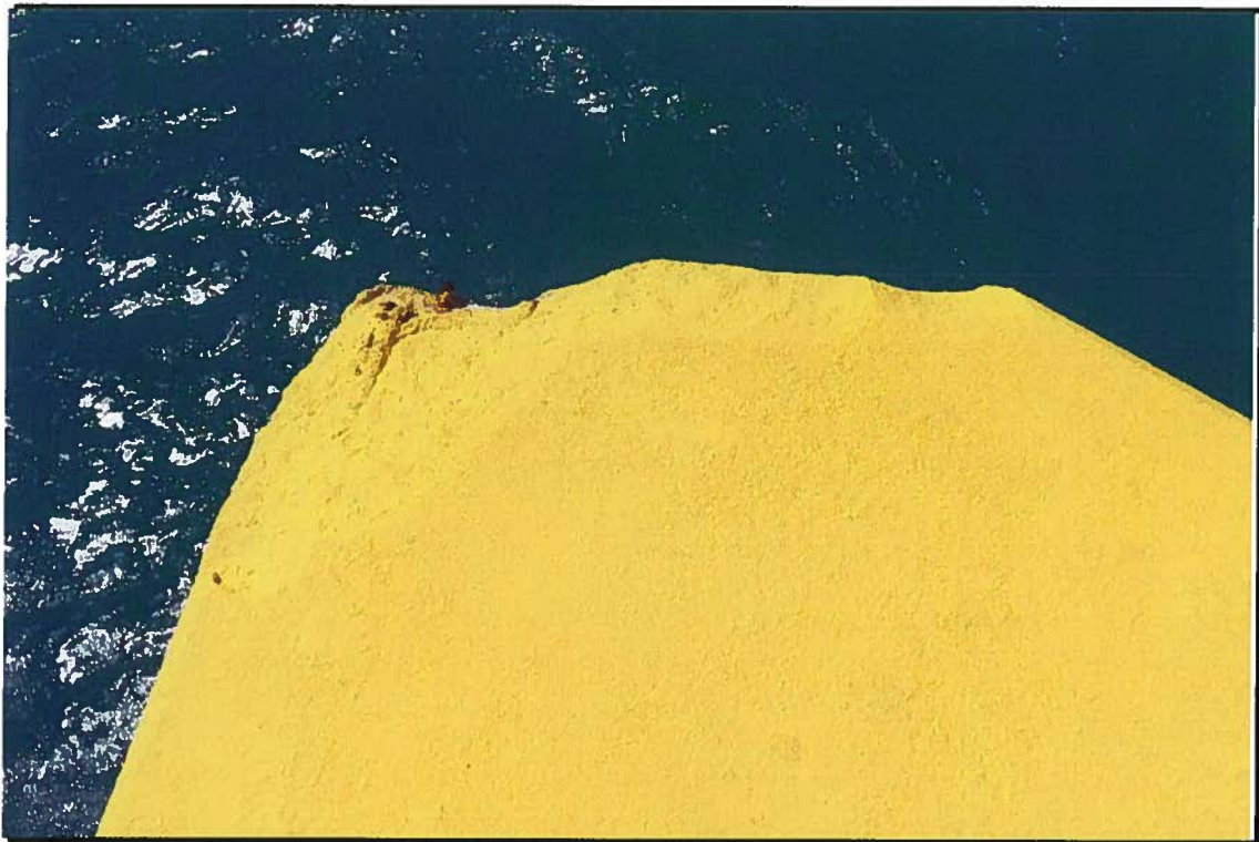
Damage to Right Side Corner Surface Deck at F-1 Dock Fender
