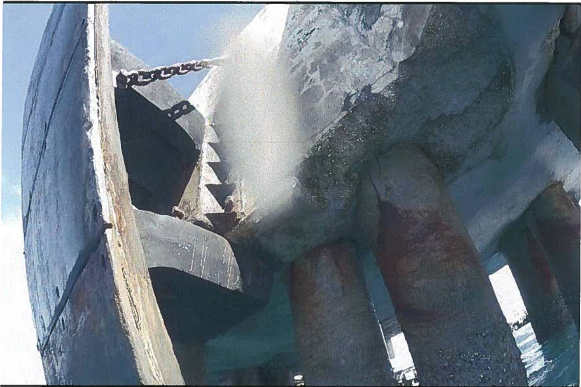
F-1 Dock Piles with Damage to Fender System and Concrete Cap
