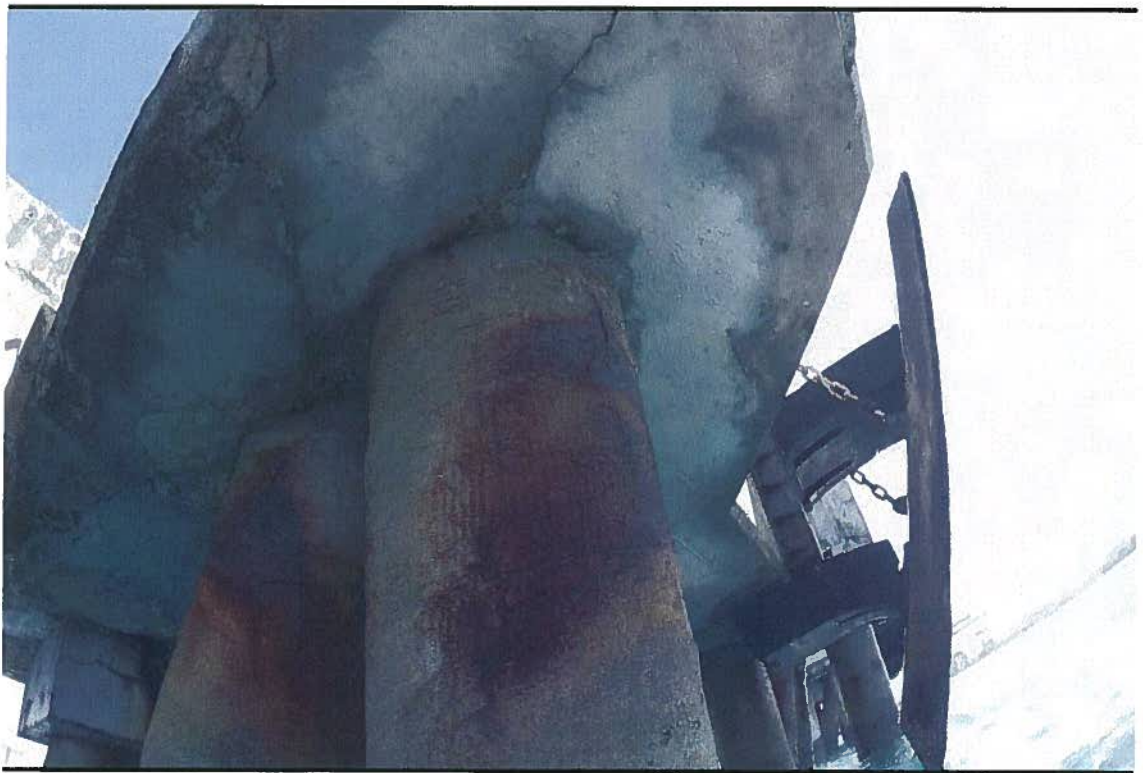
F-1 Dock Piles with Damage to Fender and Concrete Cap
