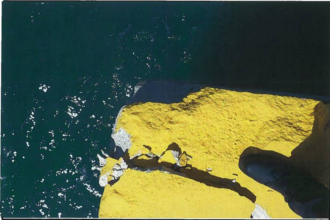
Damage to Left Side Corner Surface Deck at F-1 Dock Fender
