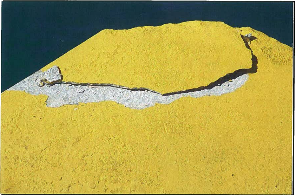
Damage to Left Side Surface Deck at F-1 Dock Fender
