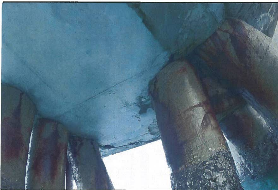
F-1 Dock Piles with Damage to Fiberglass Wrap and Concrete
