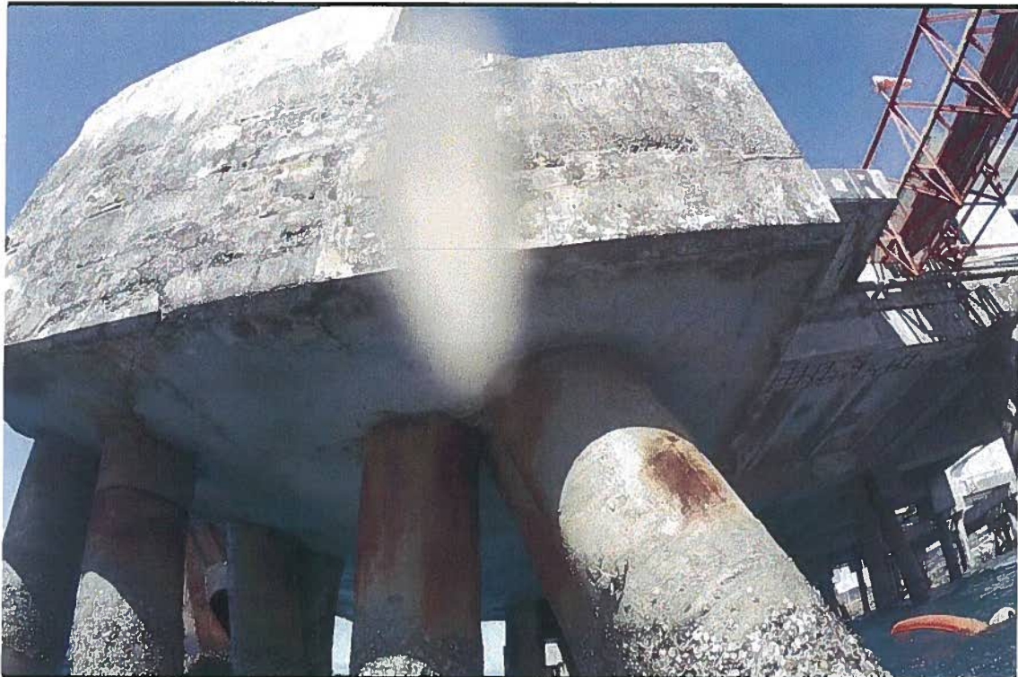
F-1 Dock Piles with Damage to Fiberglass Wrap
