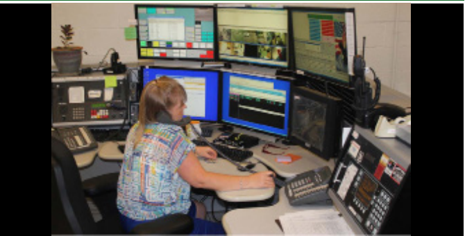
An example of an emergency communication hub.
