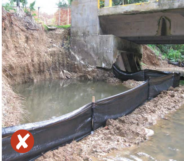
Earthen berm and silt fence do not provide adequate isolation of work area.
