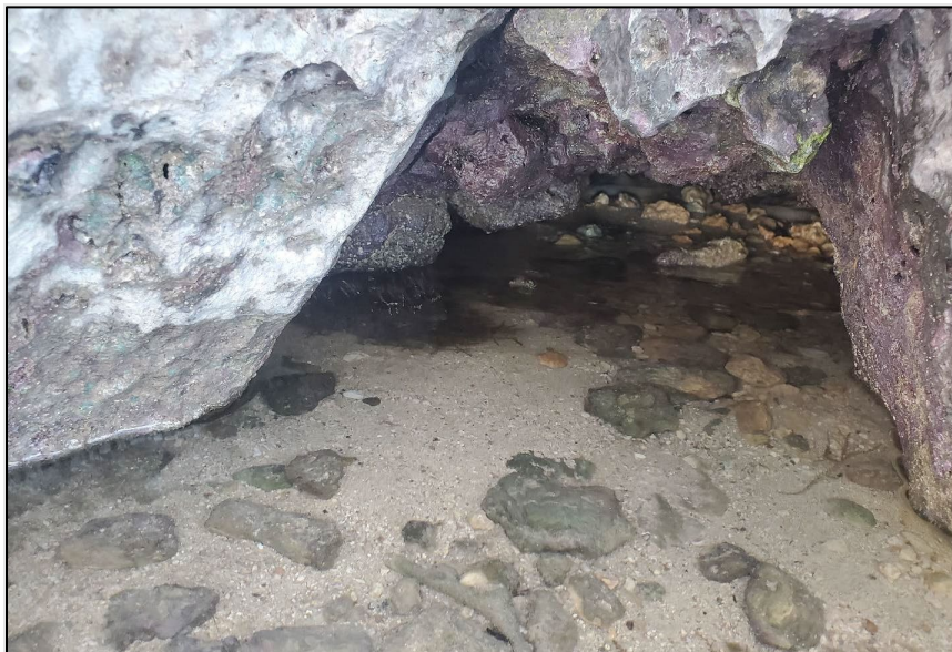
Figure 5: Close up view facing south of the undercut East Hagatna Bay seawall (USACE 2022a)
