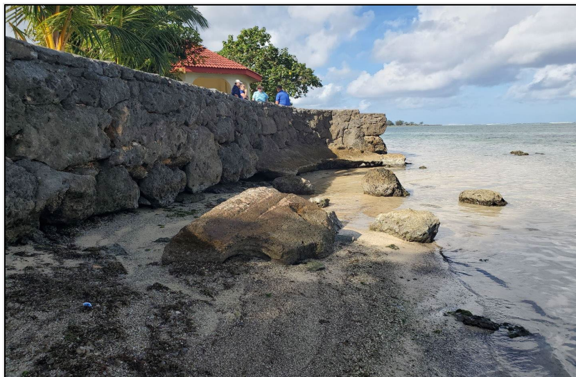
Figure 3: Existing seawall on eastern edge of Veteran's Sunset Beach Park, facing southwest (USACE 2022a). The beach has eroded below the rocks and concrete skirt, causing the seawall to crack, and undermining its structural integrity.
