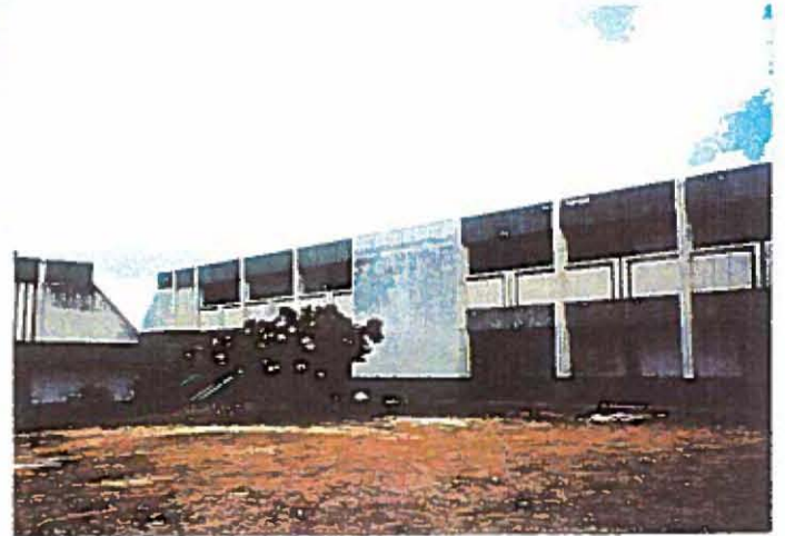
6. Building in need of paint
