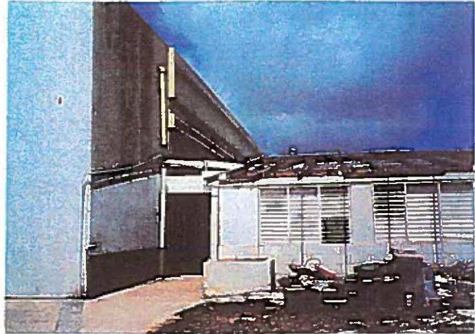
8. Rear view of gym and dilapidated industrial building
