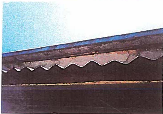
1. Cracks, chipping off roof and paint peeling on permanent structure
