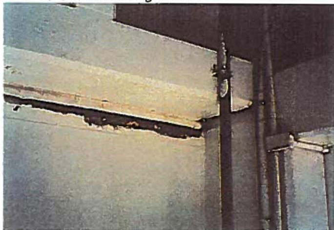
3. Exposed reinforce bars and algae growth.
