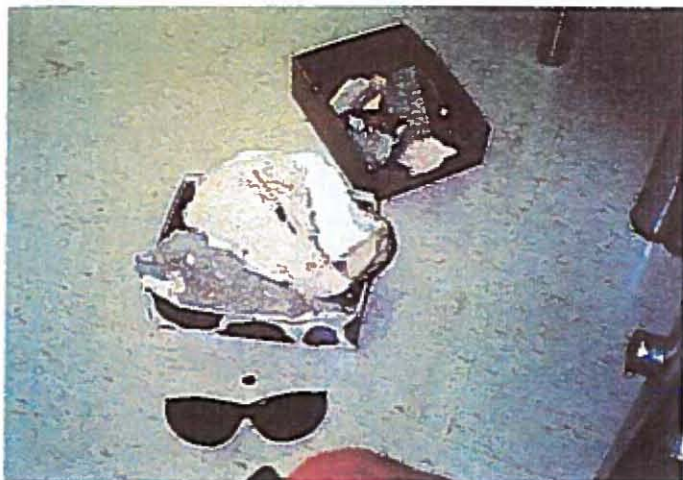
1. Chunks of falling concrete
