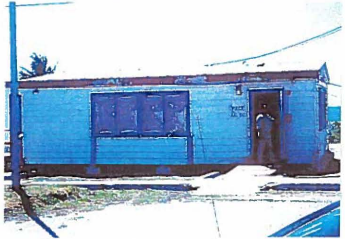
2. Unused temporary classroom termite infested
