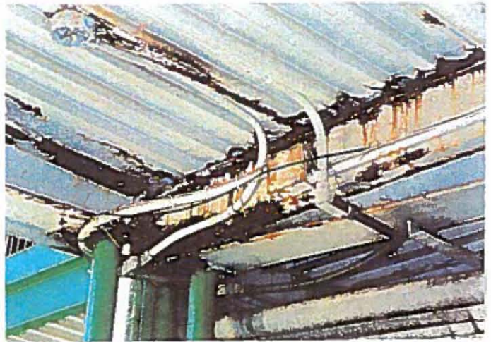
2. Corrosion of balcony in main building
