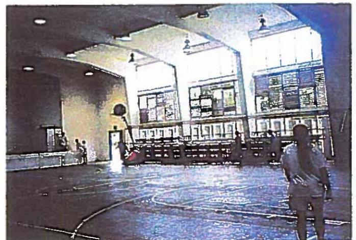
6. Broken louvers and gym bleachers in need of repair
