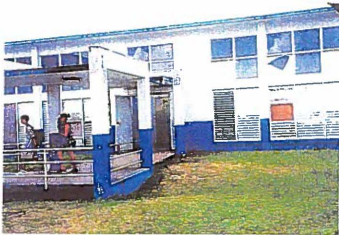
3. Broken louvers and windows flank the main building
