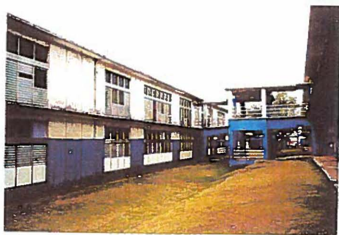
6. Peeling paint and algae covered building
