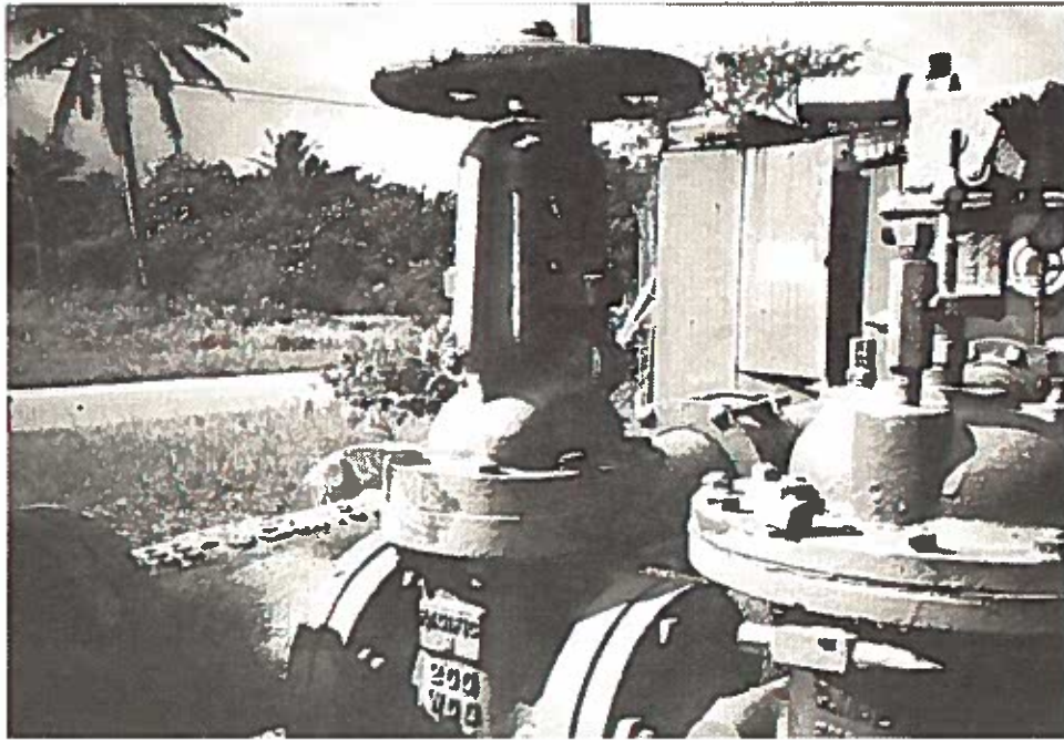
FIGURE 4-5 EFFECTS OF MARINE ENVIRONMENT ON EXPOSED PIPING
