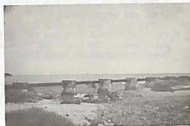
Eroded Area at Base of Gaan Point
