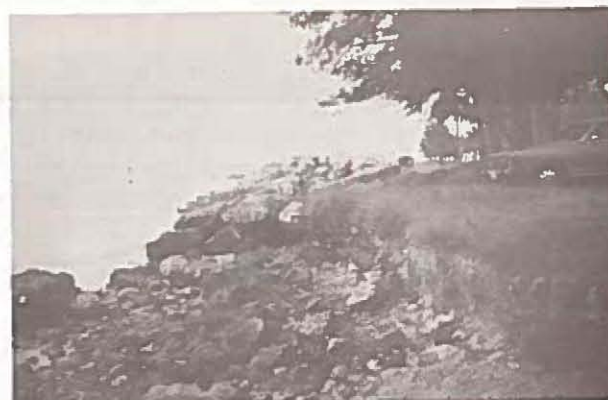
Erosion, Reach O
