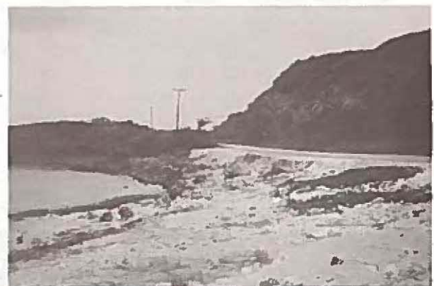
Eroding Scarp, Reach G
