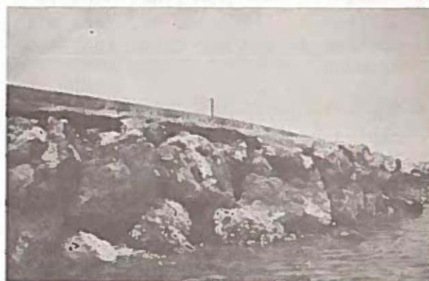
Deteriorating Revetment, Reach M
