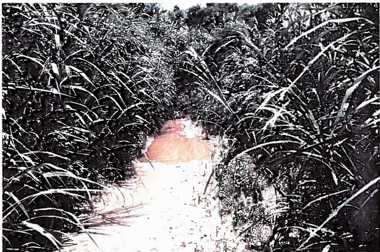
A1. Localized ponding on road in Landfill area.
