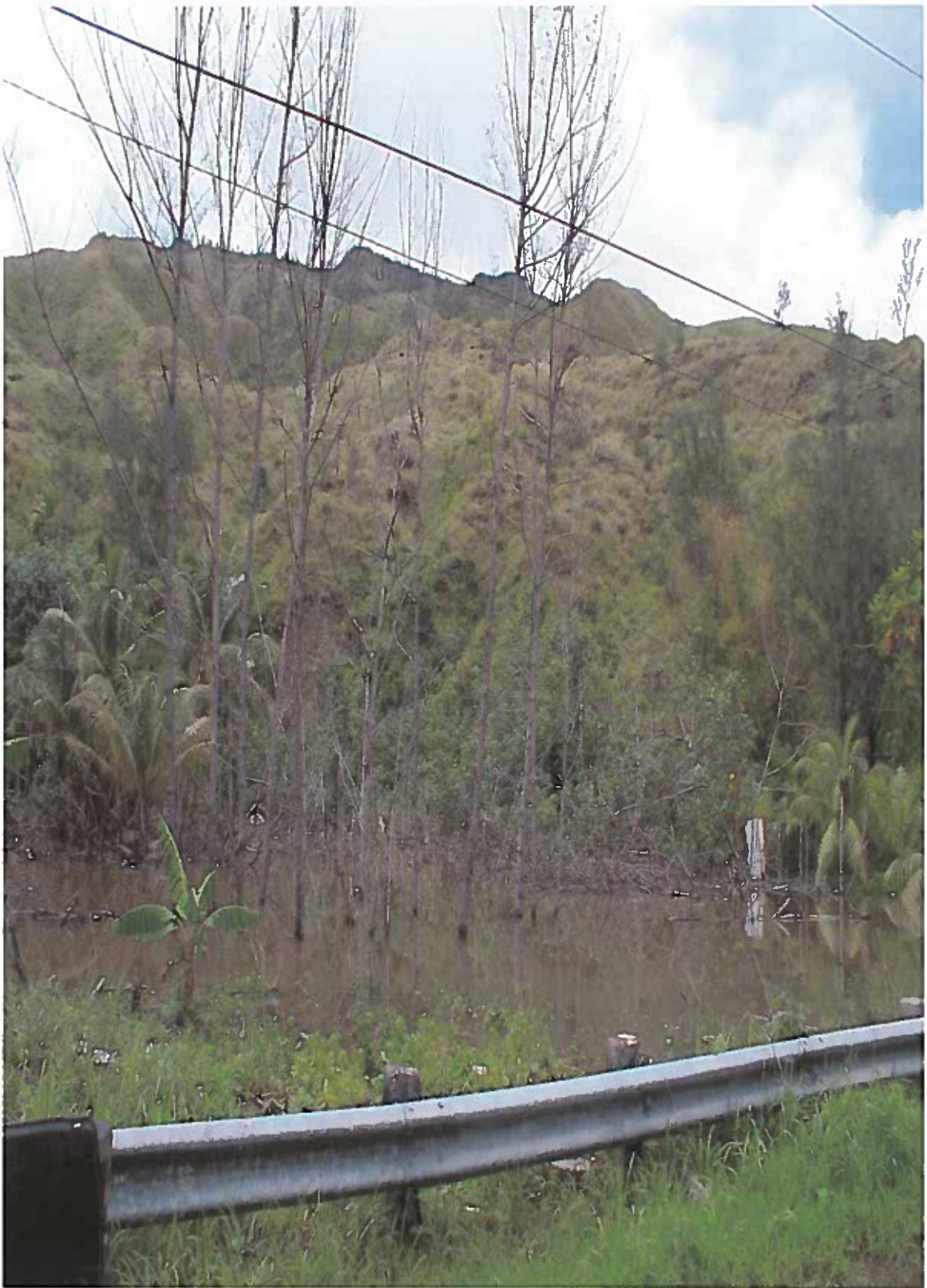
This photo was taken in front of the Agat road nearby the Cetti Bay Overlook. What should be noted from this photo is the fact that this is a 10 to 15 foot ravine area whose drainage was blocked causing the ravine to completely fill and spill over the roadside.
