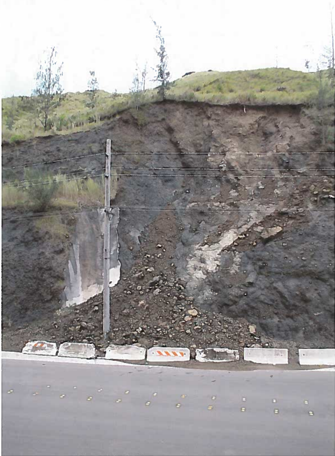
This photo was taken at the Agat – Merizo Highway. These areas normally experience landslides due to the erosion that was caused by the amount of grading during the road development.
