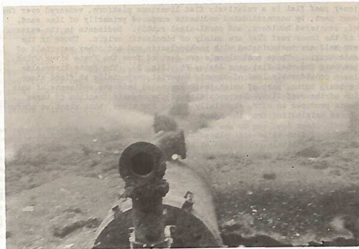
Figure 4. DIFFUSER MANIFOLD. The view here faces south and shows orientation of diffuser ports.
