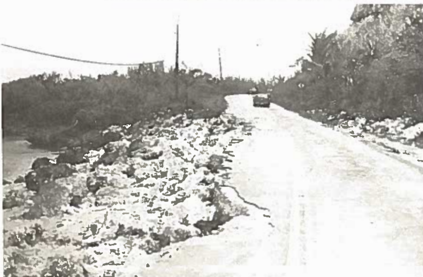
Destruction of Roads in Low-Lying Areas, Route 4
