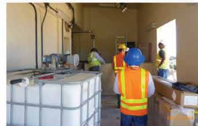
Hagåtña WWTP – Chemical mixing room
