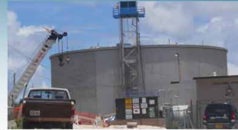
Barrigada Water Tank – Guam's first pre-stressed concrete water tank
