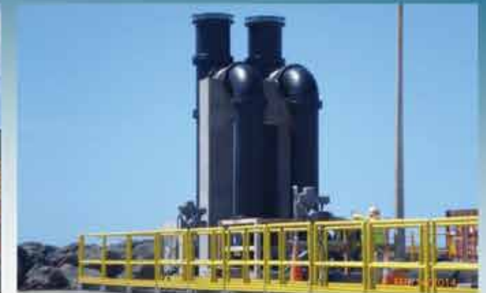
Hagåtña WWTP – New effluent vertical-turbine pumps
