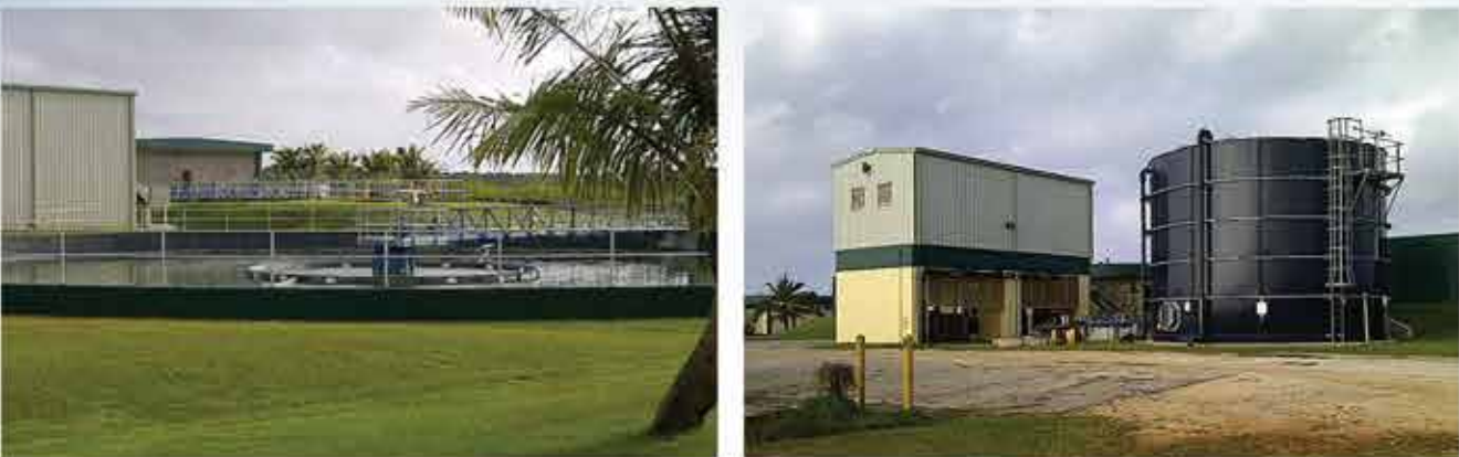
Northern District WWTP Completed Projects – Chemically Enhanced Primary Clarifiers, Sludge and Solids Handling
