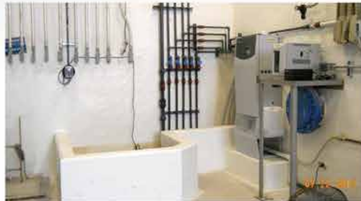
Ugum Water Treatment Plant – Total Organic Carbon Analyzer in place to monitor compliance
