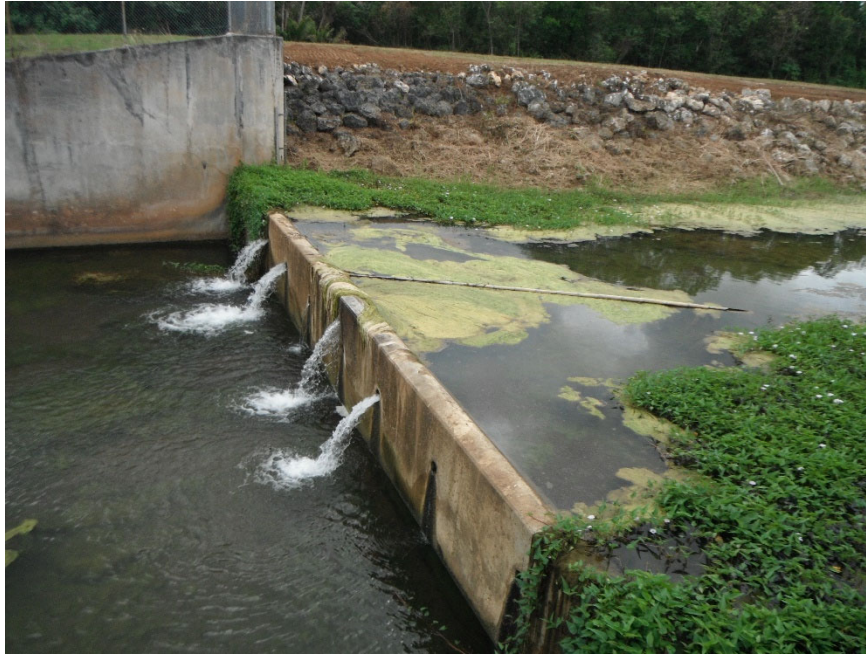
Photo 6-3: Inline Weir at Namu River FCP, Santa Rita, Guam
