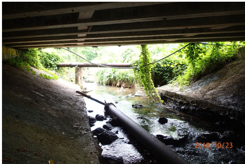
Photo 5-2: Looking downstream through the Sumay Memorial Street Bridge over Namu River at XS 1520
