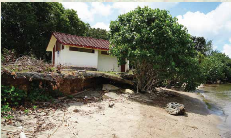
Nimitz Beach Park: Major beach erosion is pictured west of the restroom facilities. (Photo by: Guam Coastal Management Program)
